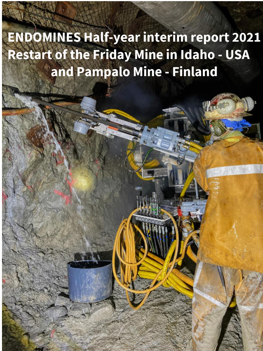
Drilling a long hole sample hole with the Boart Longyear Stopemate drill at the S4550 West Haulage – Friday Mine
